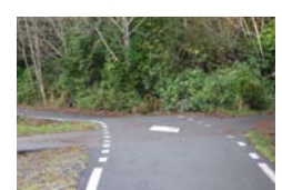
Private driveway crossings are a safety concern for MUP users.
