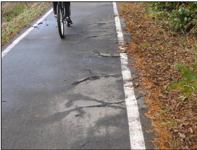
Figure 23: Tree root damage on the multi use path
