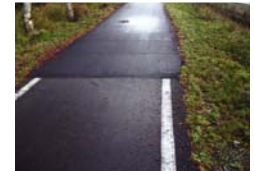
No reflective stripes in repaired area.
